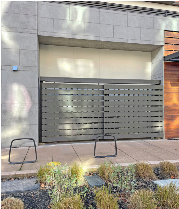
Trash collection area screened from public view by a metal gate of durable material.
