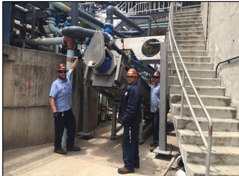
Wastewater Treatment Plant: New Hydrogritter Classifier
