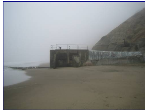
Figure ES-5 Vista Grande Outfall Located at the Beach below Fort Funston
